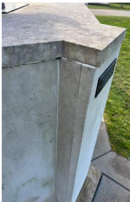
Damaged grout work
